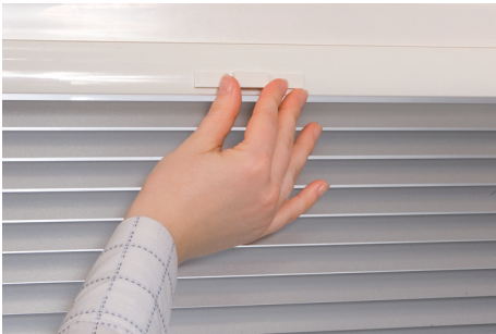
19. Check the blind operation, raise/lower and open/close is satisfactory.
